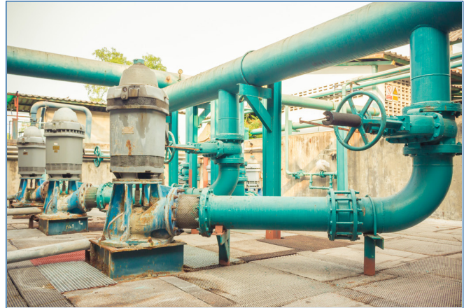
Vertical Water Pumps – pump drive and pump bearings are the components monitored. Loss of one pump could affect the ability to meet peak water demands.
