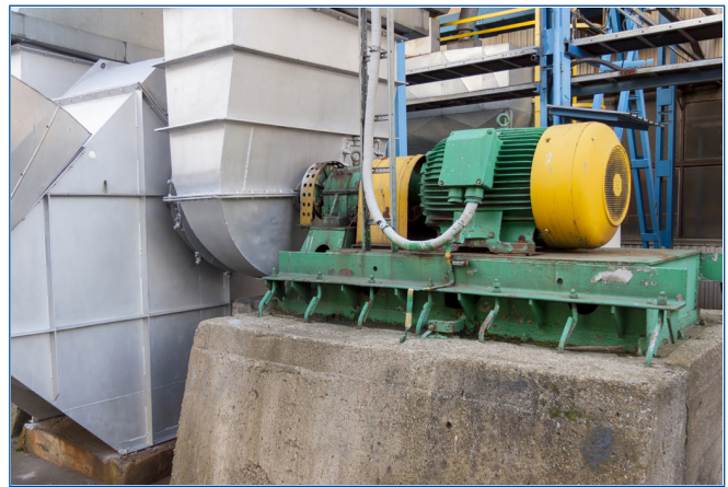
Large Centrifugal Fan – typically the fan drive and fan bearings are the components monitored. This fan does not have a backup.
