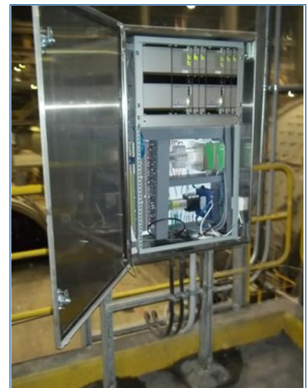
A 48-channel AMS 6500 deployed in a A6500PRE-SS-WM-IC wall mount enclosure, monitoring SAG and Ball mills at an ore processing facility.
