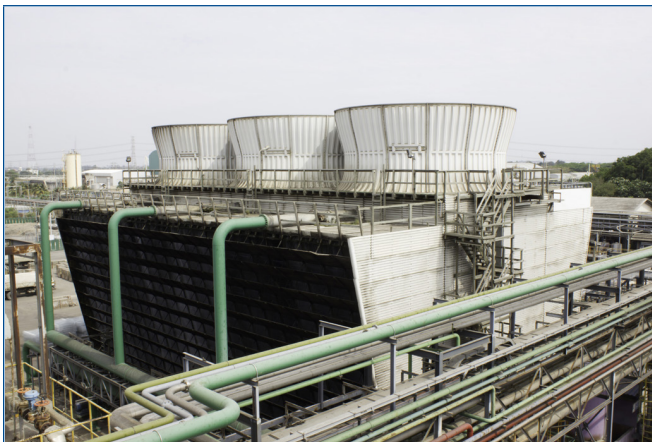
Cooling Tower Fans – typically the fan motor and gearbox are candidates for monitoring. Loss of a cooling tower fan gearbox could limit available cooling and reduce production capacity.
